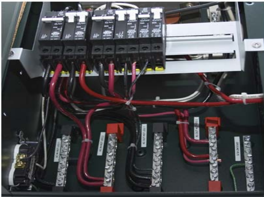
Figure 9 Picture of PS2AC wired with a fairly full compliment of breakers
