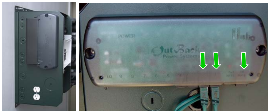
Figure 20 Mounted HUB with cover (left) & HUB connected to 2 inverters (right). The far right arrow shows where the MATE connects.
